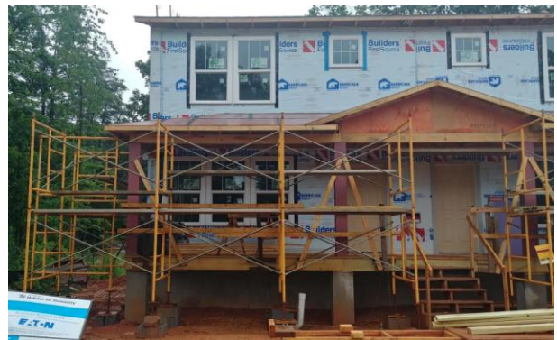
Habitat's Curry Court site will include eight two-family townhouse units like this one. One unit will be an interfaith house and Presbyterian/Methodist House #28.
